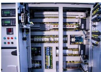
Armoires, coffrets, tableaux
